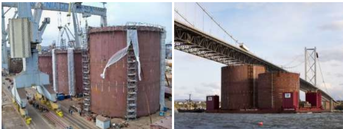
Figure 4 – Caissons during manufacture and shipping to the bridge site. (Photo: New Civil Engineer)
