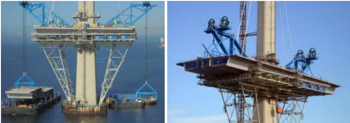
Figure 10 – First deck segment lifted by erection gantry, continuing with balanced cantilever construction.
