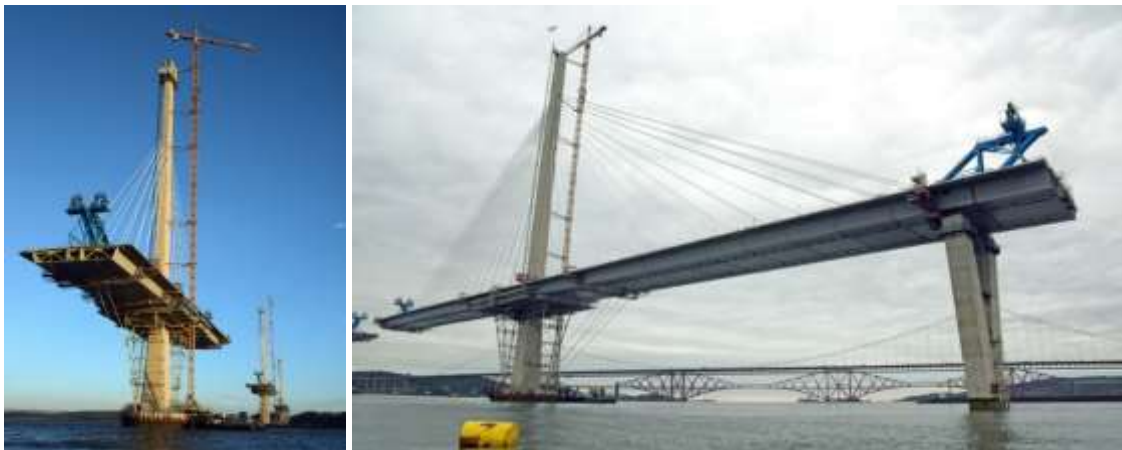
Figure 11 – Balanced cantilever erection from all towers up to the first pier pass.
